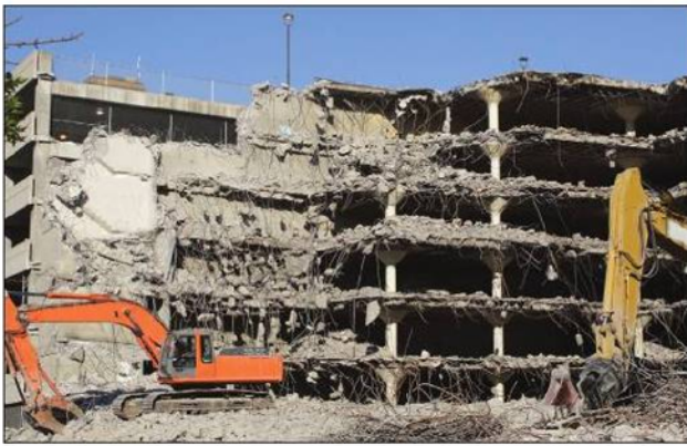
Accounting for demolition waste management and disposal is an important aspect of sustainable building.
